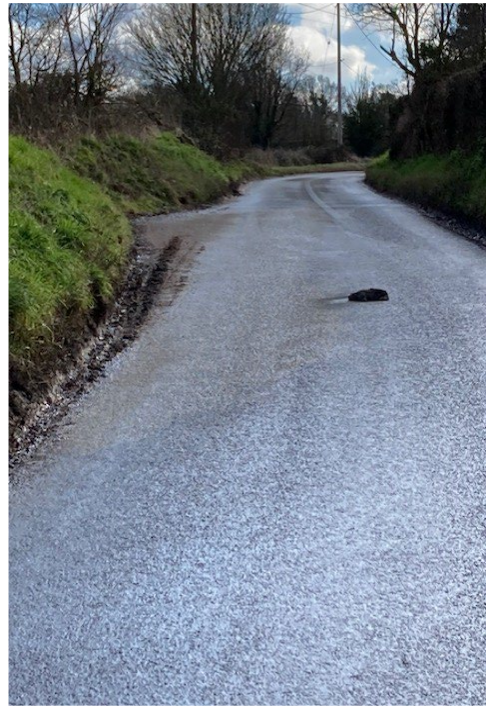
16. High sides of banks and verges showing extensive damage to land
