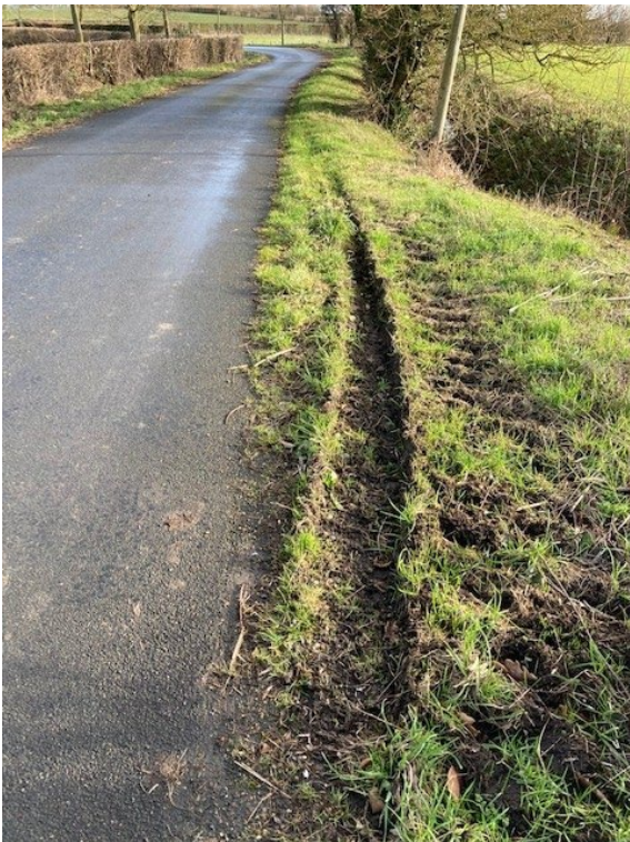
48. To show extensive damage to verges and edges caused as traffic forces a passing place
