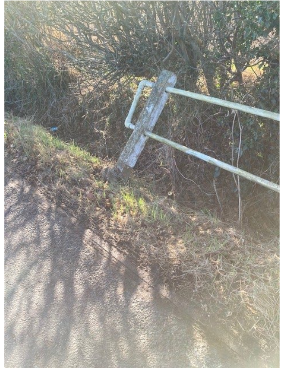
33. Damage already existing to narrow bridge
