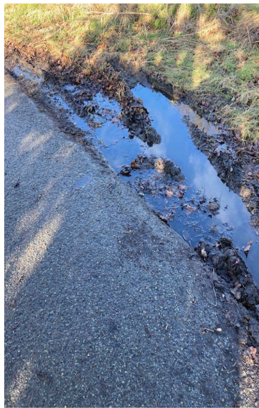
6. Extensive damage and destruction to road edge
