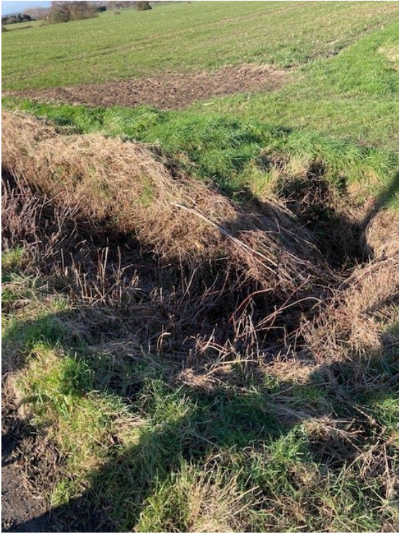
35. To show deep hidden ditches within 50cm of road edge
