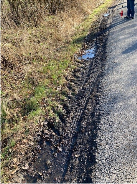
50. To show extensive damage to land and road edge. No safe haven, no passing places and no refuge point for non-vehicle road users
