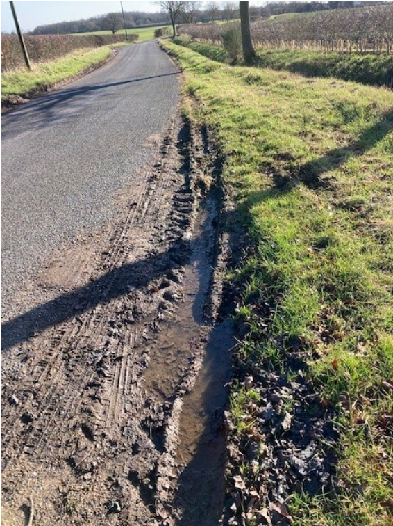
32. Extensive damage already caused by traffic forcing passing places
