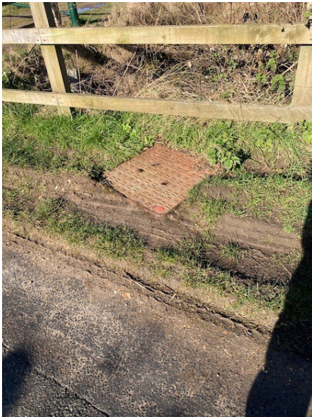
66. Raised manhole, within 25cm of road edge, already substantially damaged by existing traffic
