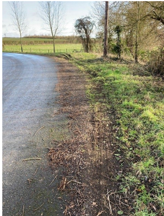
49. To show massive damage caused by existing traffic. No safe havens no pavement and no refuge
