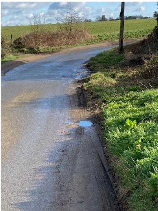
11. Blind bend and obscured vision
