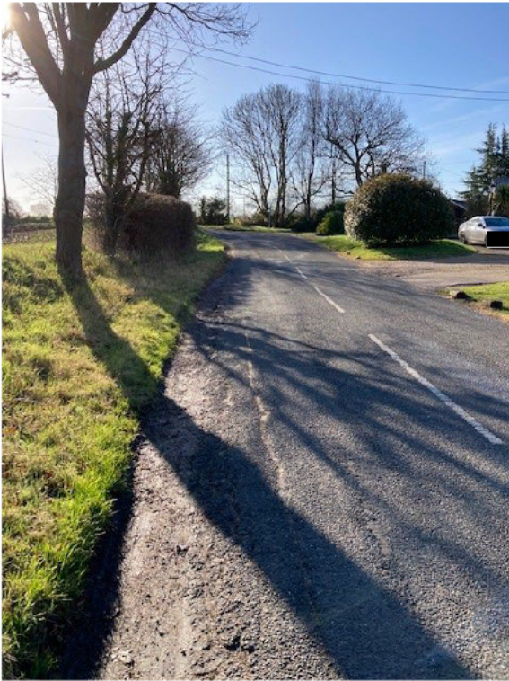
23. Extensive edge of road deterioration and damage
