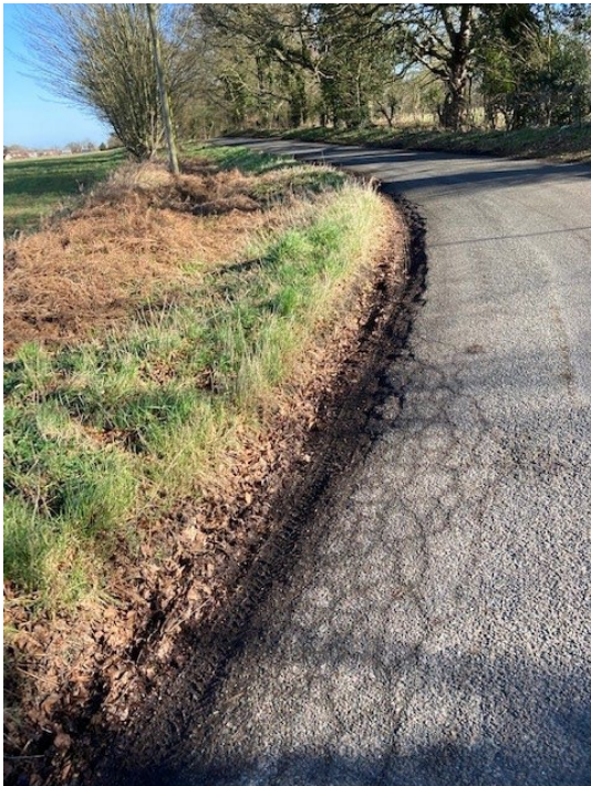
52. Showing erosion and damage to road as traffic forces a passing place
