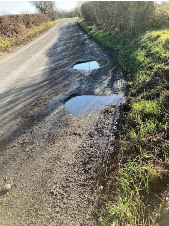
34. To show extensive verge and road edge damage
