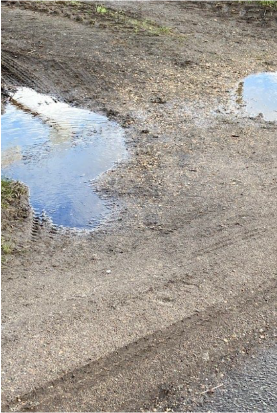
13. Further extensive damage caused by existing traffic
