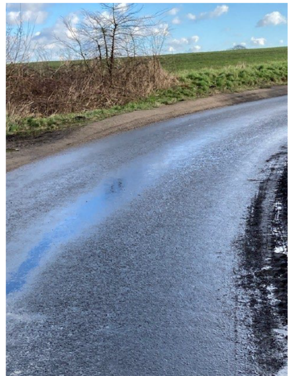
12. Road damage to high verges and blind bend
