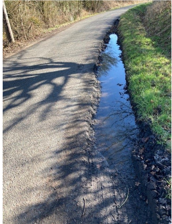
51. Showing extensive road deterioration and damage, no signage warning of school and no safe haven for pedestrians and children
